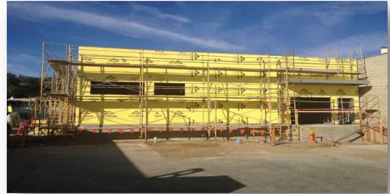
EWMS – Data Center
